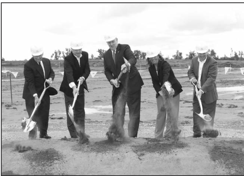
Manning the shovels at this milestone for Pioneer and the state of Missouri were from left to right: Clyde M. Hawes, Presiding Commissioner, New Madrid County; Paul Schickler, President, Pioneer Hi-Bred; Jay Nixon, Governor of Missouri; Jo Ann Emerson, U.S. Representative and Alejandro Munoz, Vice President, North America, Pioneer Hi-Bred
